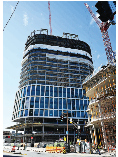
At a topping-off ceremony in September, Samuels & Assoc. marked the completion of vertical framing for an office and life science tower anchored by CarGurus’ headquarters on Massachusetts Turnpike air rights parcel 12. Photo courtesy of Samuels & Assoc.
